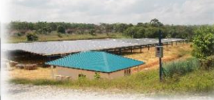
Professional services for Grid-Connected PV Inverter Site Testing and Power Quality.
